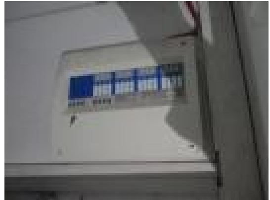
Panel of fire alarm system.JPG
